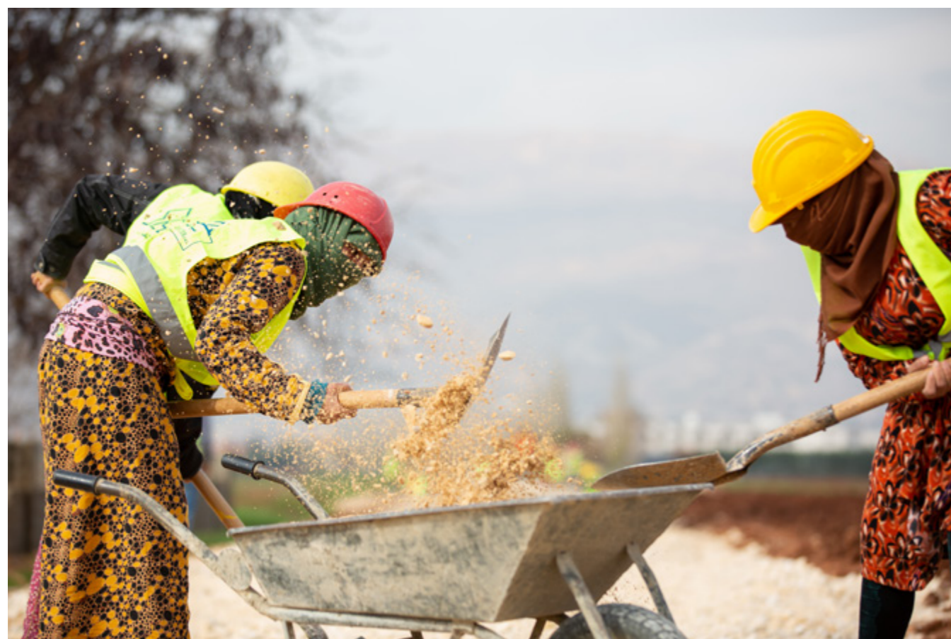
Rehabilitation of over 14 km of agricultural roads benefitting 700 farmers & their families in East Zahleh. UNDP Lebanon, 2019.
