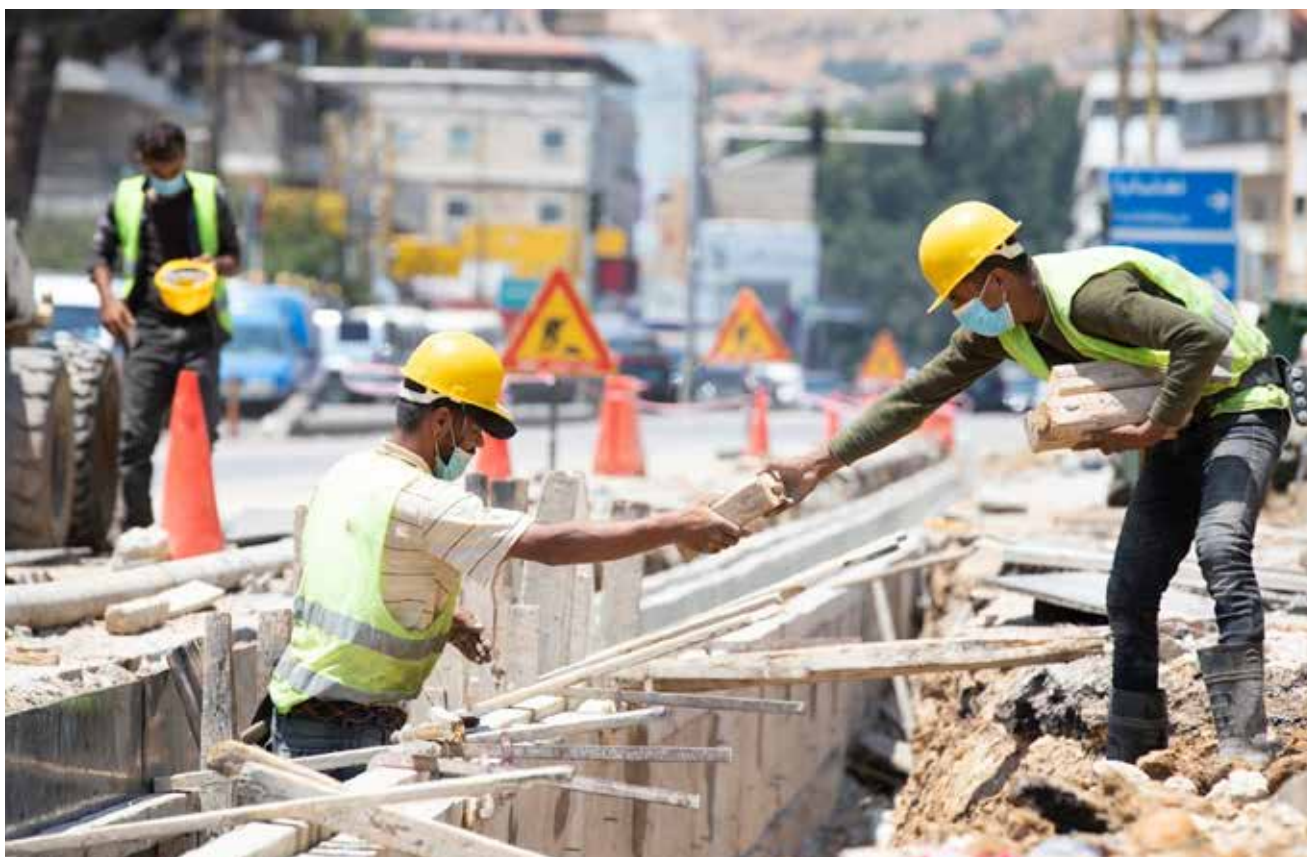
Construction of stormwater canals in Chtoura prevent cross-contamination and flooding during heavy rains.
