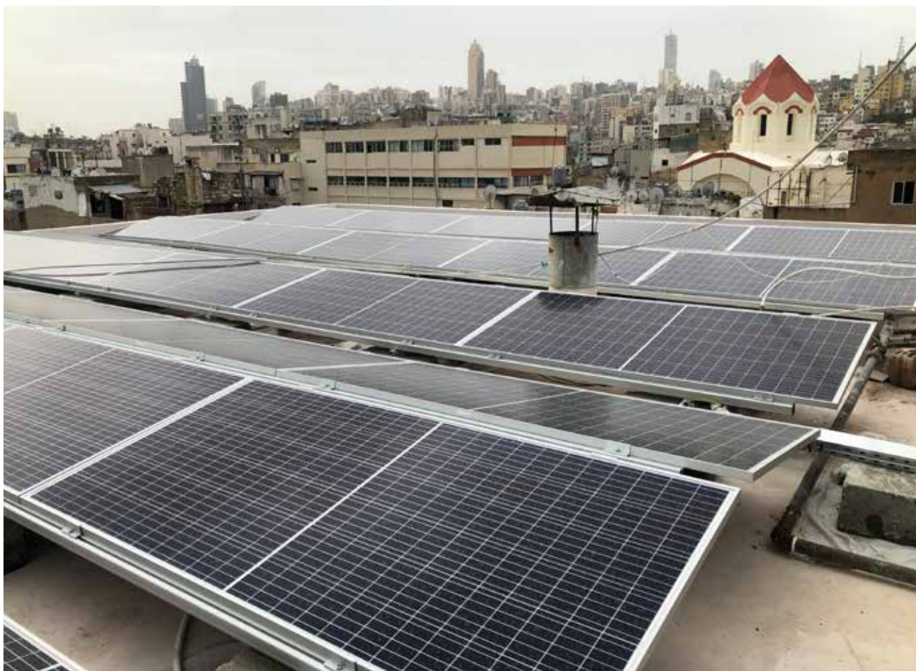
Solar panels installed on the roof of the community centre in Maraach, Bourj Hammoud
