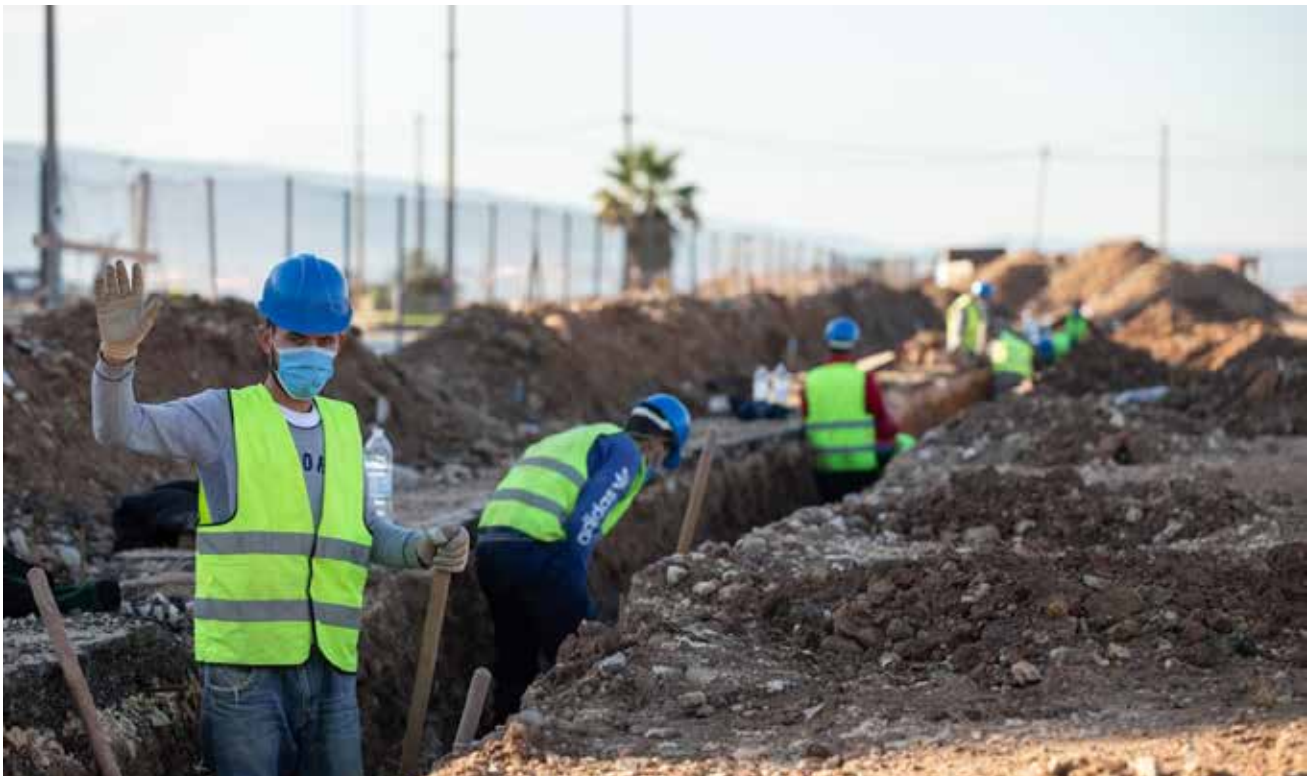
The rehabilitation of Tripoli's Al Mina Corniche is providing workers with job opportunities, improving the infrastructure and enhancing touristic and economic activity.
